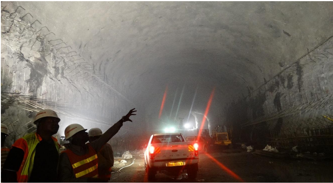
Fig. 13: MEMD and UEGCL Officers inspecting the anchoring of the Crane beam in the underground power house
