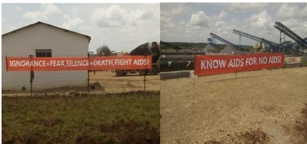
Figure 64: HIV/AIDS awareness material placed at different sites in Isimba Hydropower Project Areas in Kayunga
