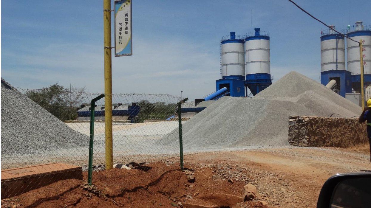
Figure 14: The Batching Plant on the left bank of the river was completed and is operating
