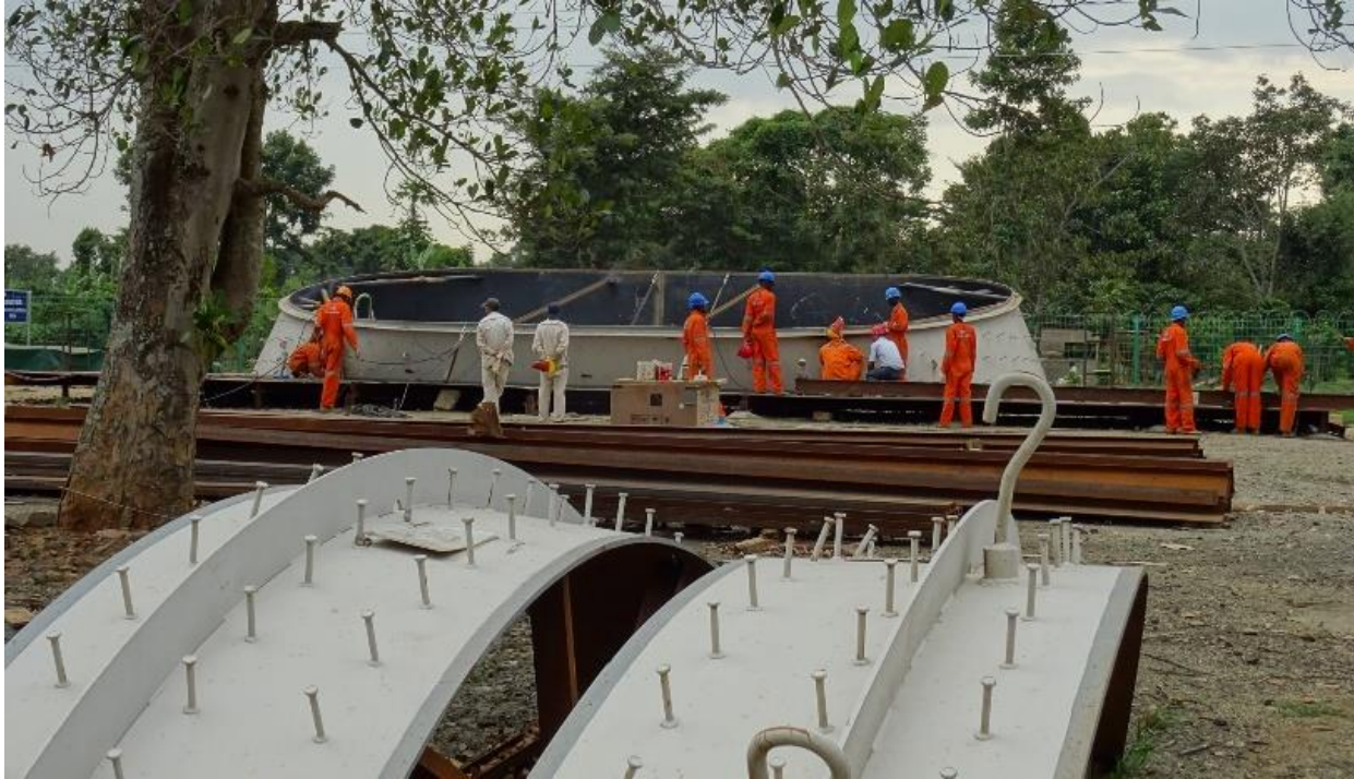
Fig. 16: CWE staff assembling the spiral casing formwork and draft tube embedded parts (September 2015) at Isimba HPP
