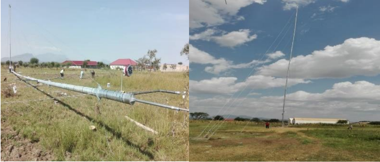
Fig. 21: A set of two wind measuring equipment installed at Napak and Kotido District headquarters
