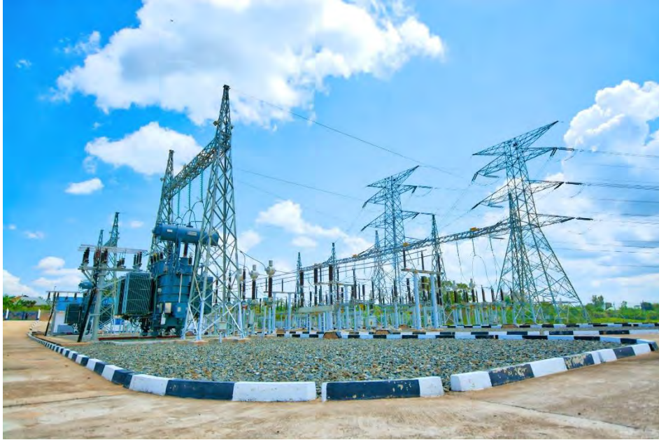
Picture 4: New Fort Portal Substation
