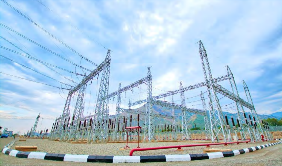
Picture 6: New Nkenda Substation
