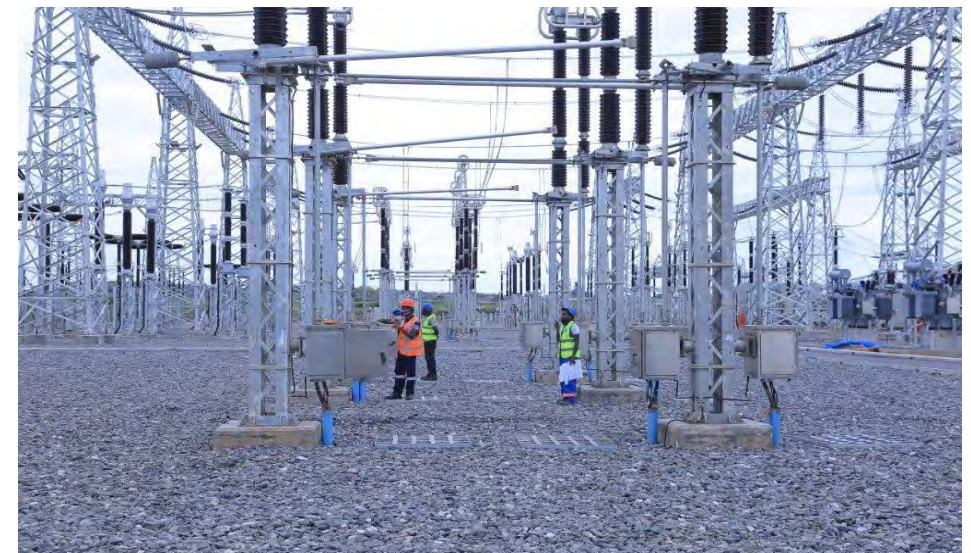
Picture 7: Karuma Switchyard precommissioning tests
