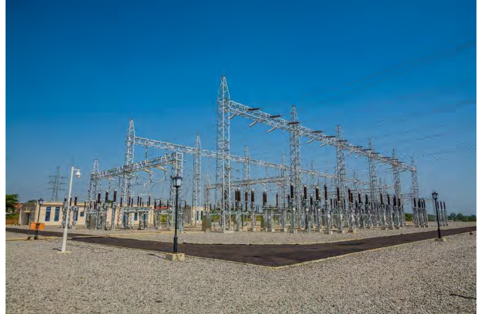
Picture 9: Isimba HPP Switchyard
