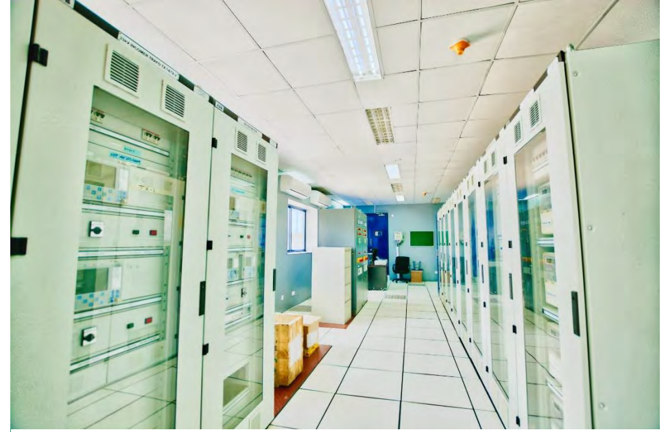
Picture 5: New Fort Portal Substation Control room
