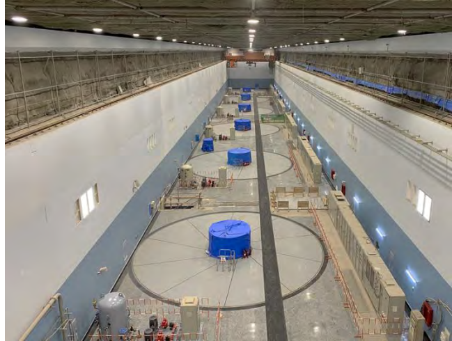
Picture 1: An aerial view of the machine floor at the 600MW Karuma Hydropower Plant.
